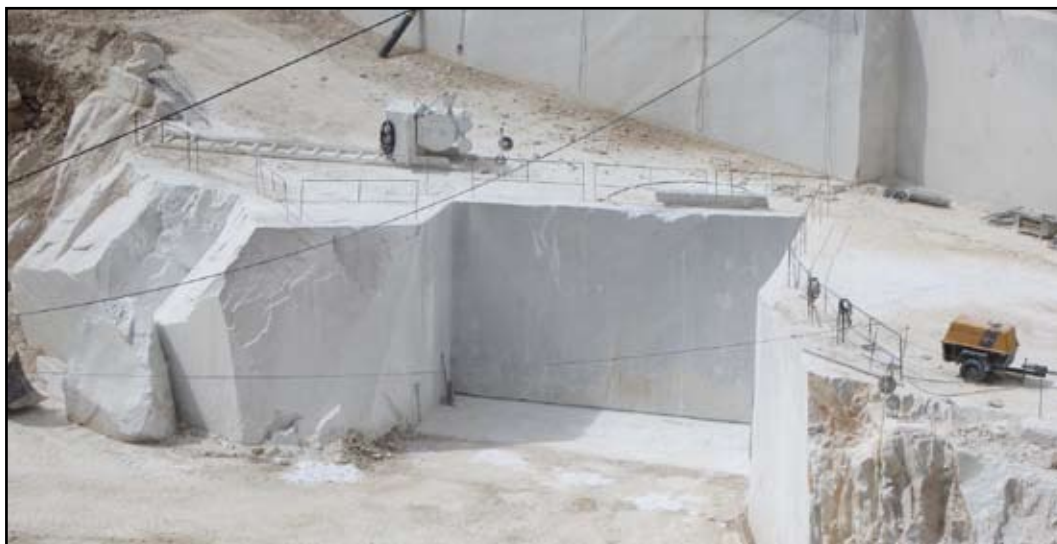
Figure 7. A recent image of a bench currently being worked in the Crestola quarry, with faces that have been cut by crawler-mounted chain-saws.
